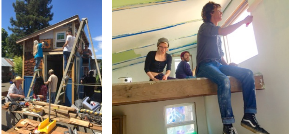
Figure 7. Left: Completing the exterior of the second tiny house. Right: Repainting the interior.
