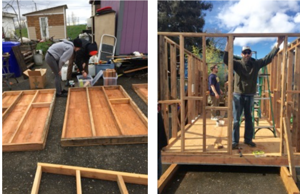
Figure 5. Left: Wall sections were built in the ReBuilding Center workshop and then transported to Dignity Village for assembly. Right: The pre-fab wall sections were not square enough, and were disassembled and the framing completed without the plywood already attached.
