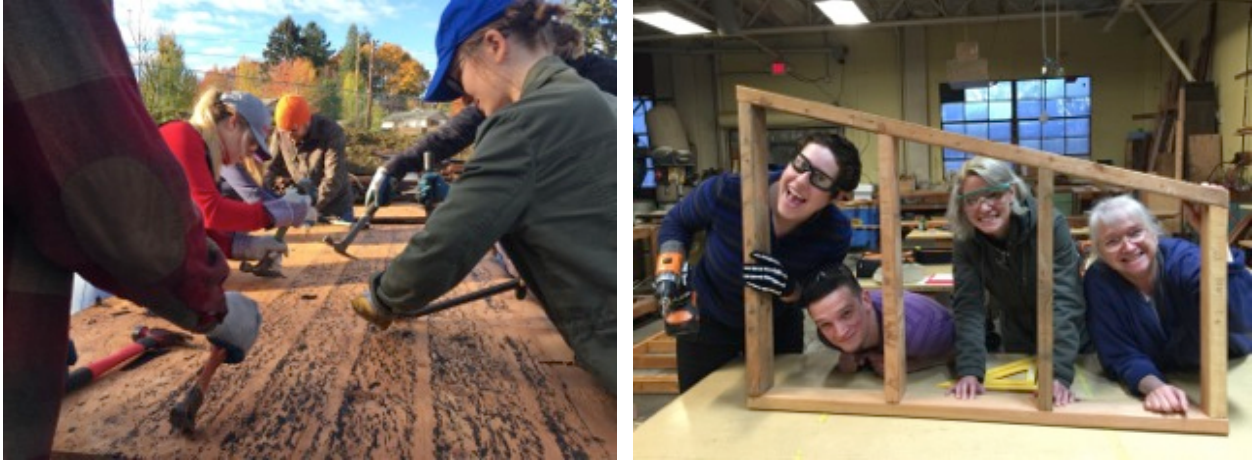
Figure 4. Left: De-nailing the plywood at the ReBuilding Center secondary site. Right: Building the wall sections in the workshop provided by the ReBuilding Center.
