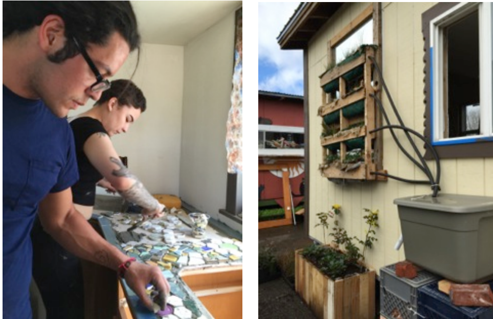
Figure 2. Left: Building a reclaimed broken-tile countertop for the kitchen. Right: A greywater system using native Oregon plants for the kitchen sink.
